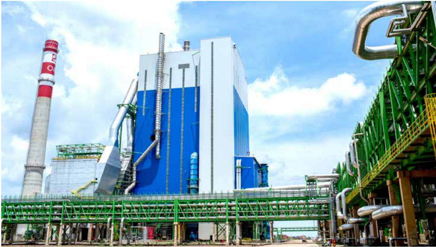
Recovery boiler, generating renewable energy Recovery boiler, menghasilkan energi terbarukan
